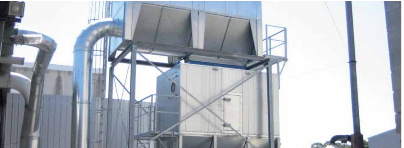
Midwesco Filter Resources, Nordic Air Filtration and TDC Filter's filtration solutions are installed worldwide
